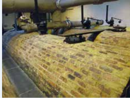
The boilers viewed from their rear
