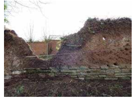
A section of wall prior to repairs (image courtesy of Nottinghamshire County Council)
