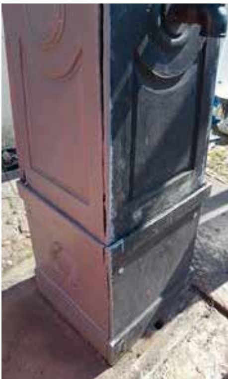
The primer was applied once the panels had been fixed back into position
