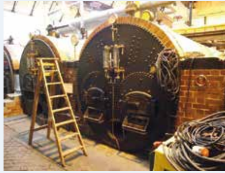
The Lancashire Boilers
