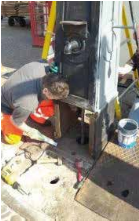
Day 1 of the restoration, note the soakaway located beneath the trough and the absence of any pump machinery
