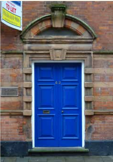
Partial Gibbs Surround at 42 Kirkgate. Note that the lower sections of the surround have been removed
